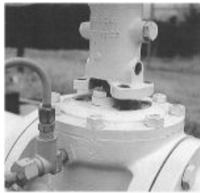
PACKING GLAND BOLTS EXPOSED
